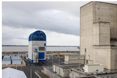
Figure: Ultimate emergency diesel generators have to be secured against extrem temperatures – on the site of the Blayais power plant (Gironde) by Florence Levillain /Signatures /Médiathèque IRSN
